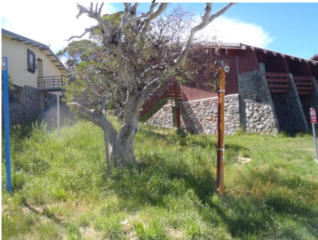
Figure 13: Photo of the fire hydrant on the eastern side of Plum Pine Road
