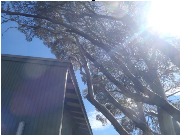
Figure 7: Photo of the existing tree overhanging lodge on the south-eastern corner - recommended to be trimmed
